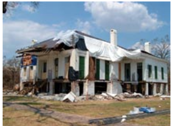
The folks who built Beauvoir knew a little bit about hurricane-resistant housing it seems... The last home of Jefferson Davis survived the past 120 years, including "Camille" and now "Katrina." Other buildings on the site were not so fortunate.
