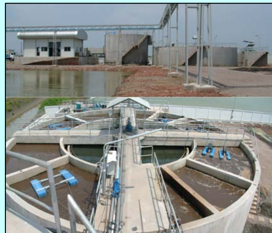
Food Processing Wastewater Treatment Plant
