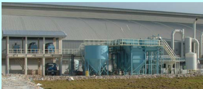
Inclined Plate Clarifier in Ceramic's Wastewater treatment Plant
